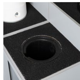
4. Empty socket is a potential trip hazard
