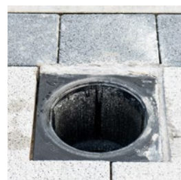
4. Empty socket is a potential trip hazard
