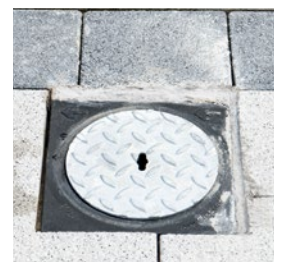
5. Blanking plate removes hazard
